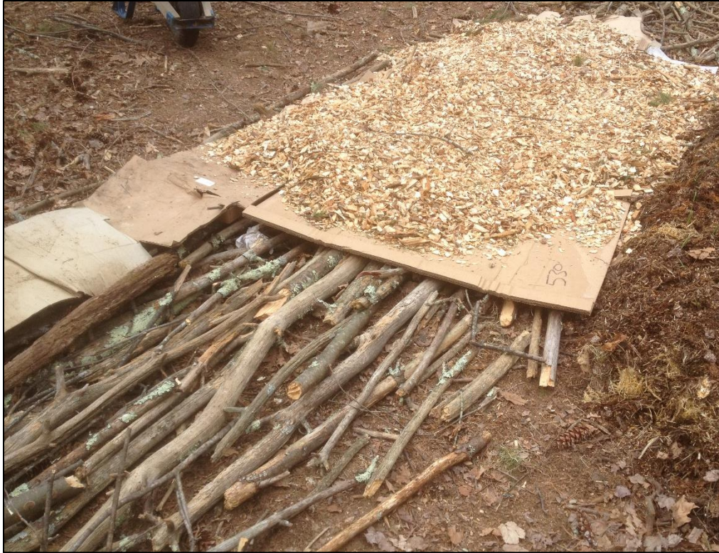
Building up above wet spots with brush, rotted wood, cardboard and woodchips
