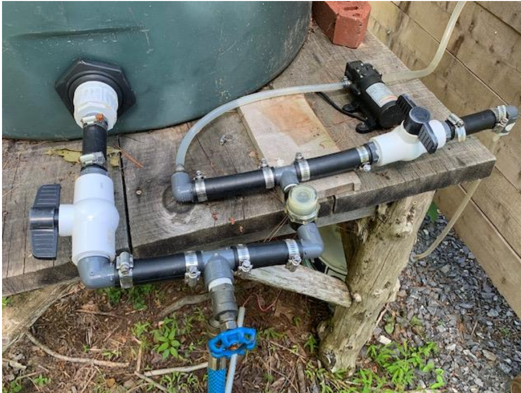
A storage tank with a garden hose adapter, an inline screen filter, a drinking water adapter and a 12 volt pump for added pressure.
